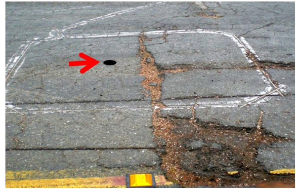
Figure 2: Photo showing WVDS installation within a failed inductive loop in very poor pavement
